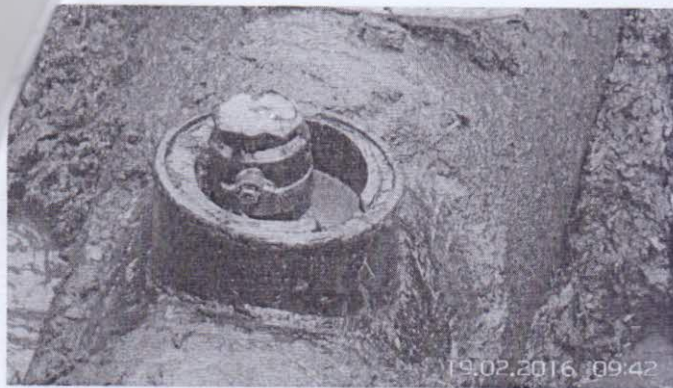
Figure 1: 2 Inch Valve that was previously conned.
